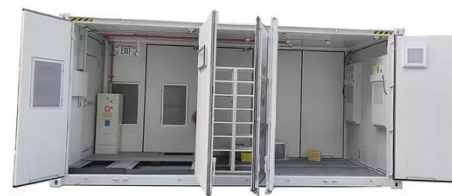
1075KW HH ESS
